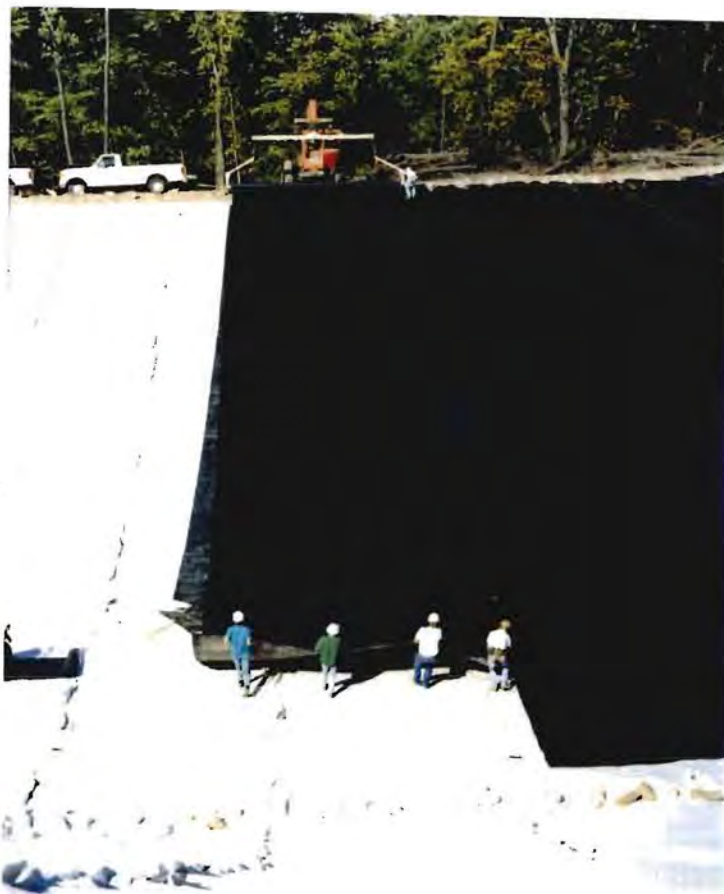
Photo No. 6: (17-18 September 1996) Placement of the primary geomembrane over the geocomposite leak detection layer.
