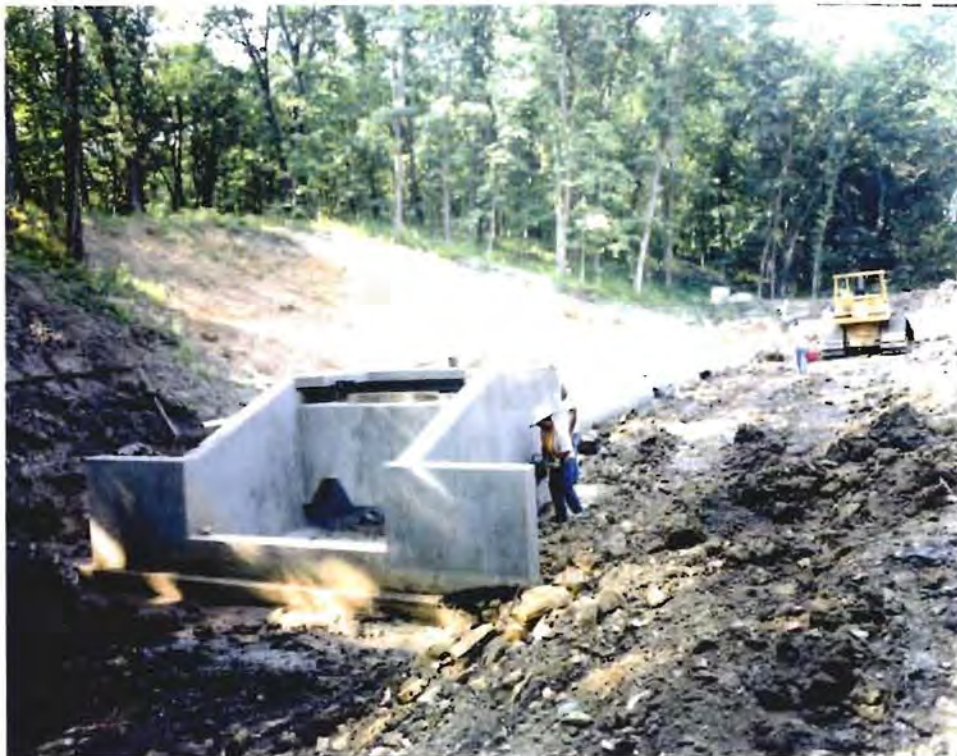
Photo No. 6: (14-15 August 1996) Construction of the stilling basin and outlet works conduit is complete. Compaction of the soil immediately adjacent to the structures is in progress.
