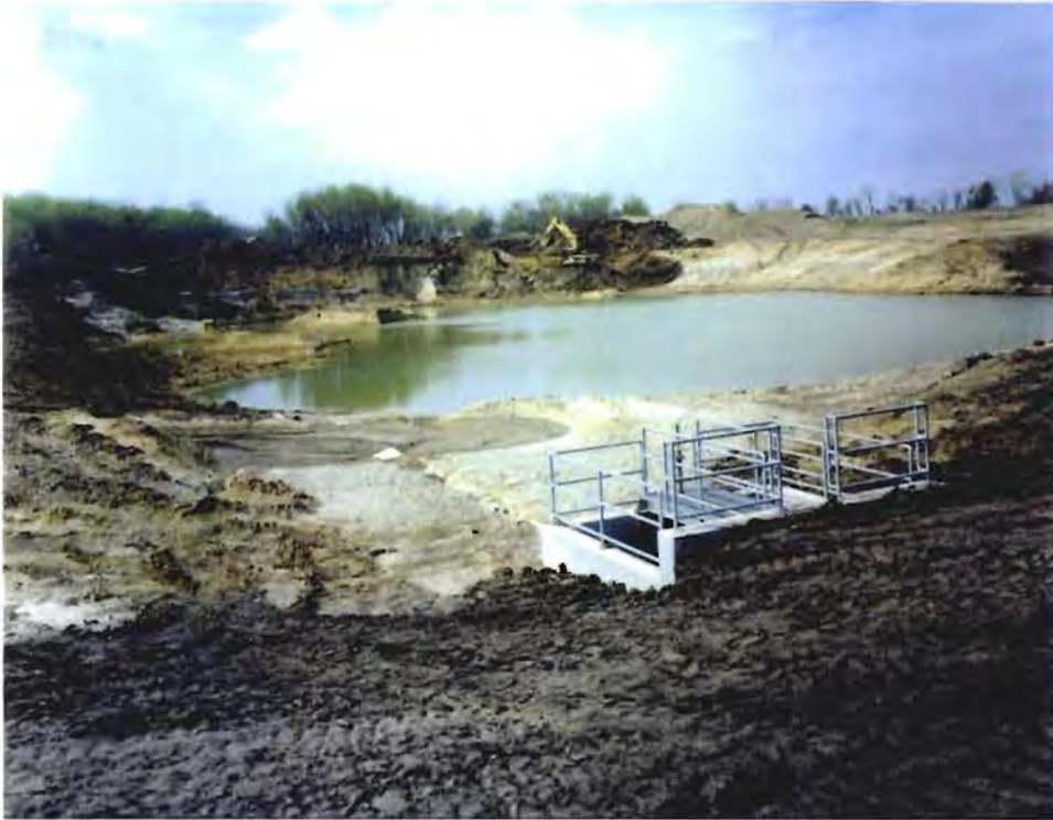
Photo No. 9: (29 April 1997) View of the completed intake structure. Note the excavation of borrow material in the background.
