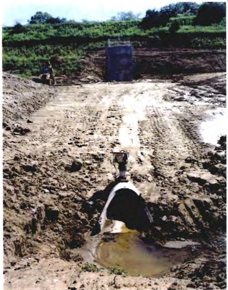
Photo No. 11: (6 August 1997) View of the inlet to the intake structure-low level intake pipe.
