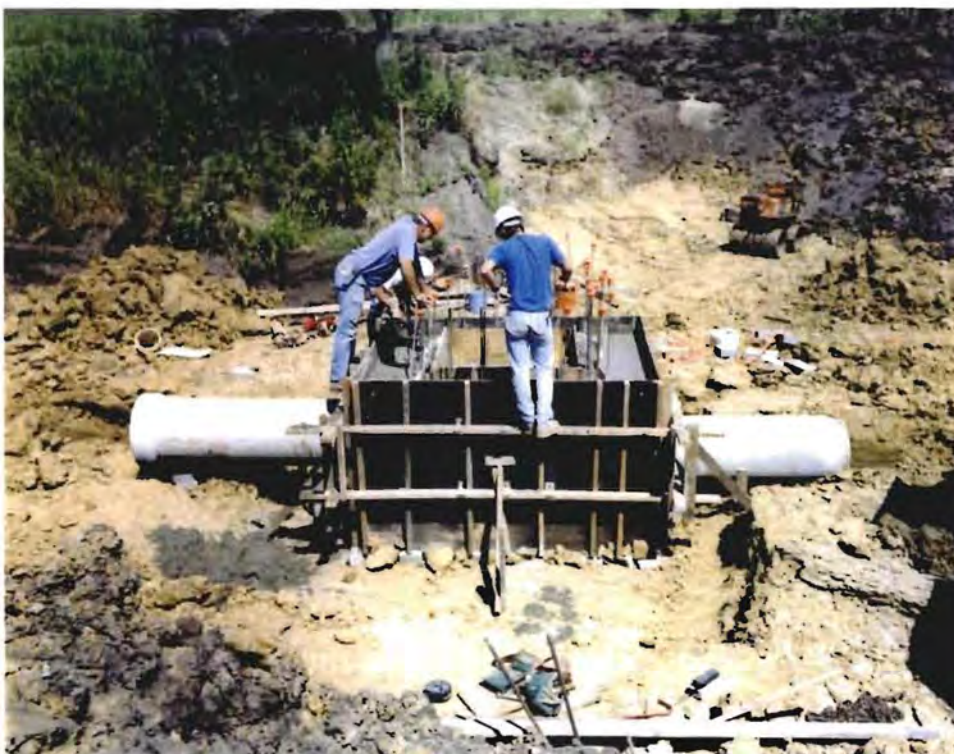
Photo No. 12: (6 August 1997) Looking northeast at the gatewell and outlet works for the upstream wetlands hydraulic control structure.
