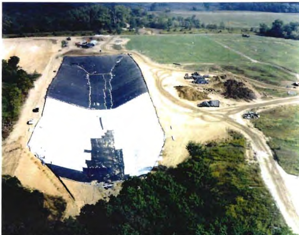
Photo No. 5: (17-18 Sept 1996) Looking north at the Trench 6 Soils Repository under construction at the IDA. The Inert Landfill is in the right of the photograph.
