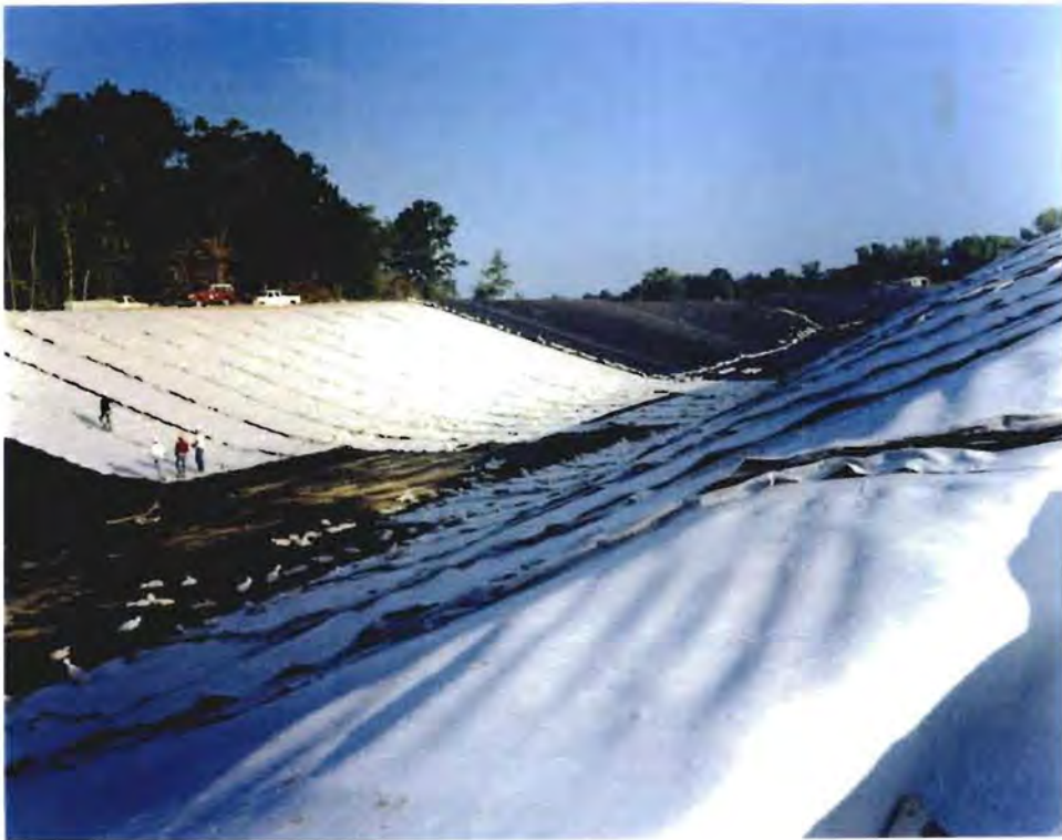
Photo No. 7: (17-18 September 1996) View of the progression of geosynthetic placement. Visible layers include the secondary geomembrane, the geocomposite leak detection layer, and the primary geomembrane.
