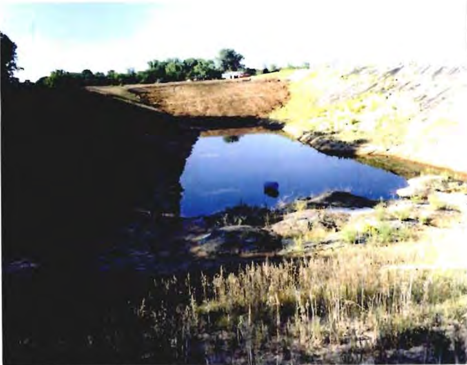
Photo No. 15: (6 August 1997) View of Trench 6, looking north. On this date, approximately 13,300 cubic yards of contaminated soil had been placed into the cell. The soil contains approximately 14,300 pounds of explosives.
