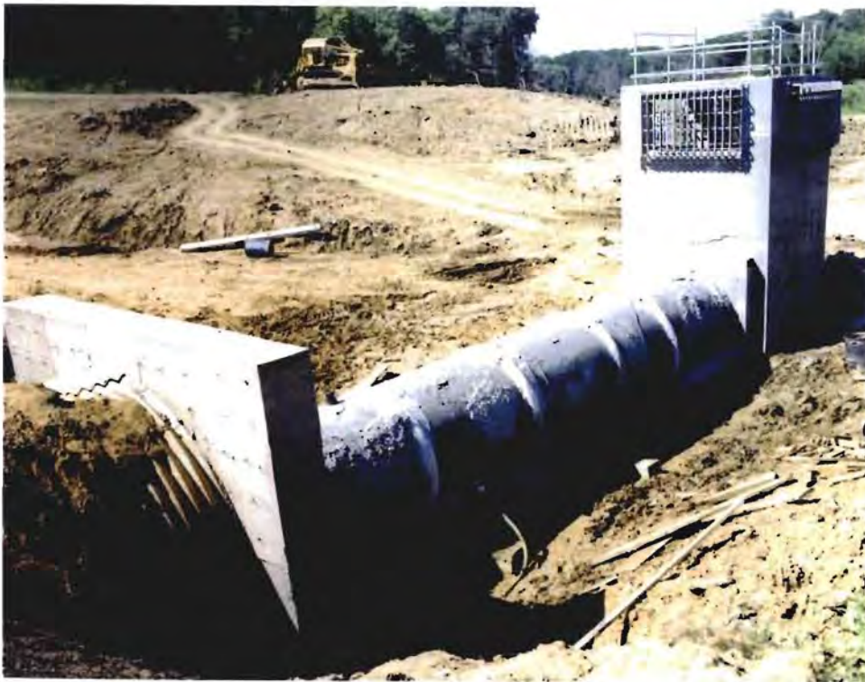
Photo No. 10: (6 August 1997) View of the completed intake structure, newly constructed portion of the outlet works conduit, the plug wall, and the existing railroad embankment conduit.
