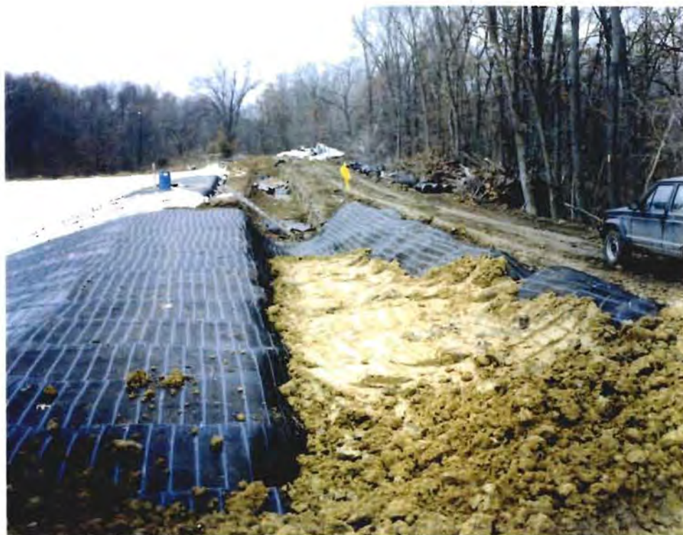
Photo No. 10: (19 November 1996) View of the geogrid anchor trench along the west side of Trench 6. Note the smaller geosynthetic anchor trench in the background.
