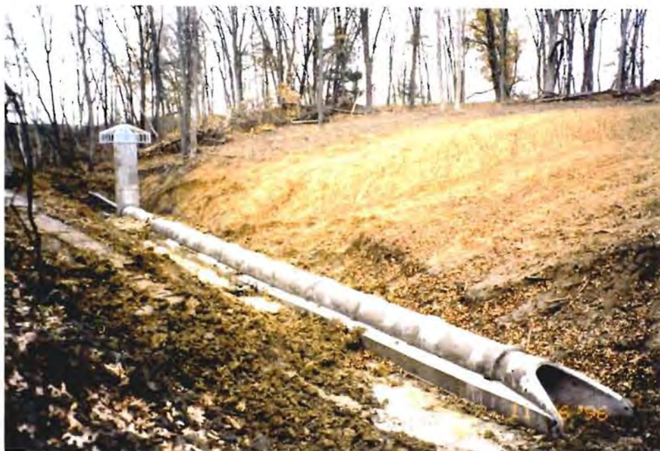
Photo No. 3: (6 November 1996) View of the completed intake structure and outlet works conduit, prior to construction of the embankment.
