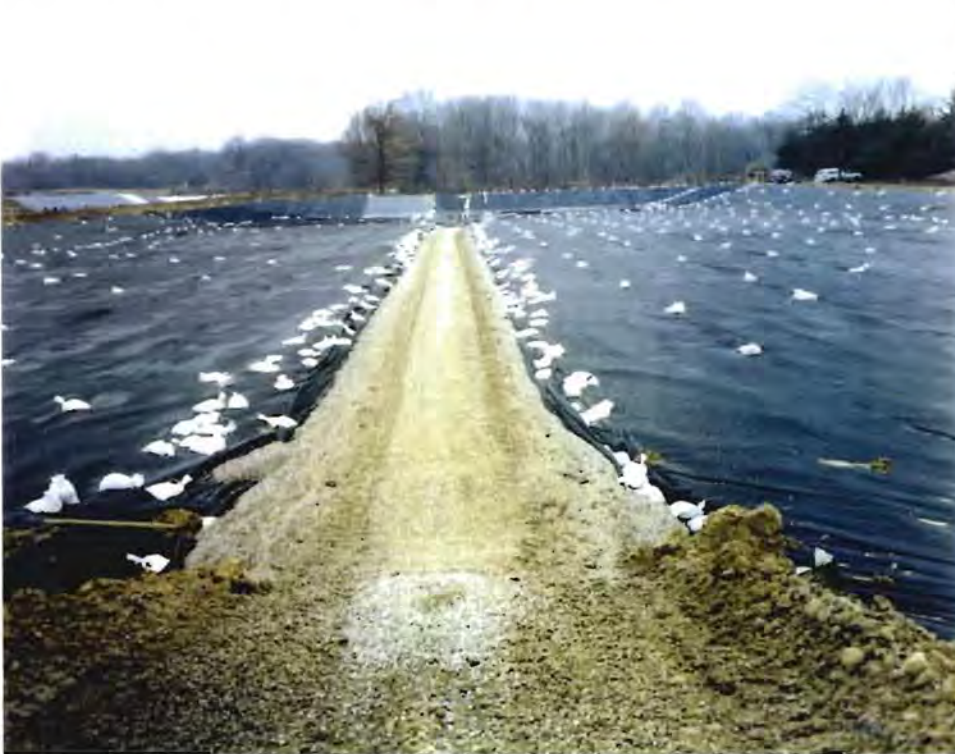
Photo No. 6: (19 November 1996) The bottom liner system is nearly complete. Following the installation of a filtration geotextile, the CAMU will be able ready to receive contaminated soils.
