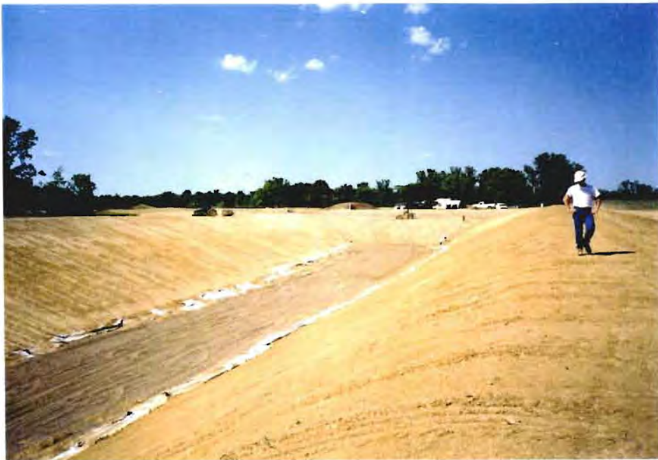
Photo No. 3: (8 August 1996) Initial grading is complete. The geocomposite and pea gravel seepage collection layers are complete at the bottom of the trench.
