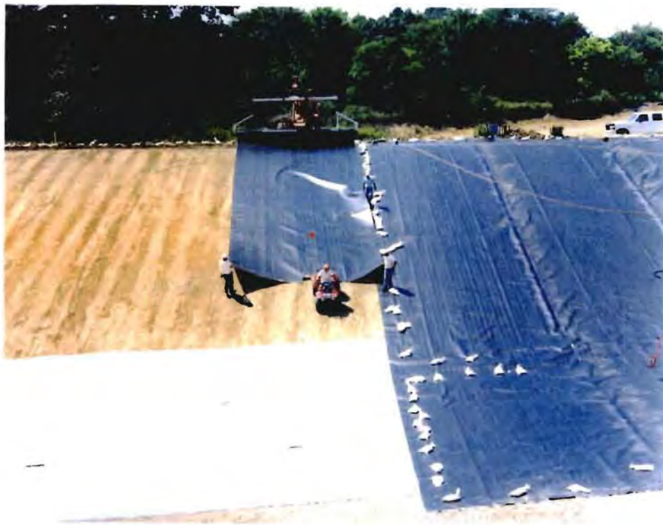
Photo No. 5: (14-15 August 1996) Placement of the secondary geomembrane liner on the west sideslope of the trench.
