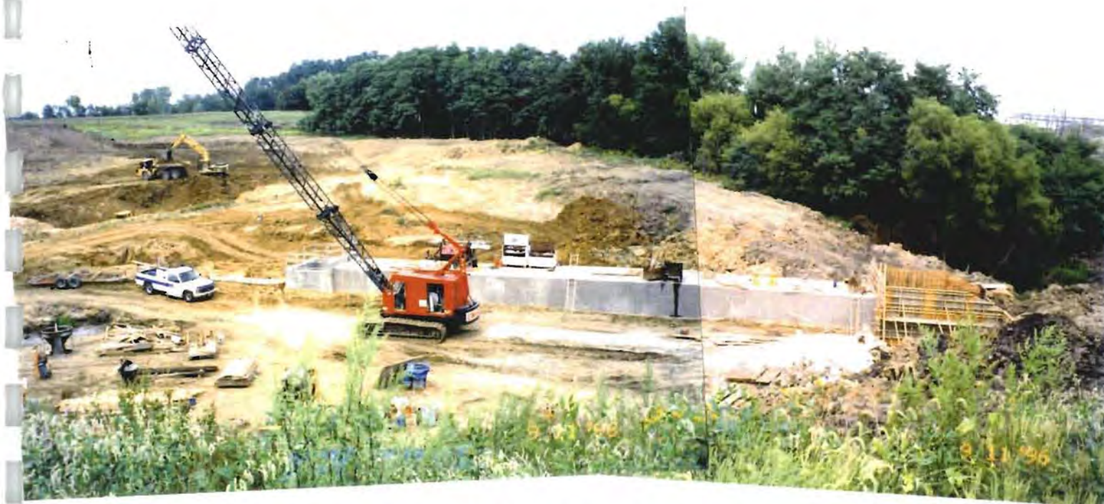
Photo No. 4: (11 September 1996) The intake structure, low level intake, and outlet works conduit are complete. The stilling basin is currently under construction.
