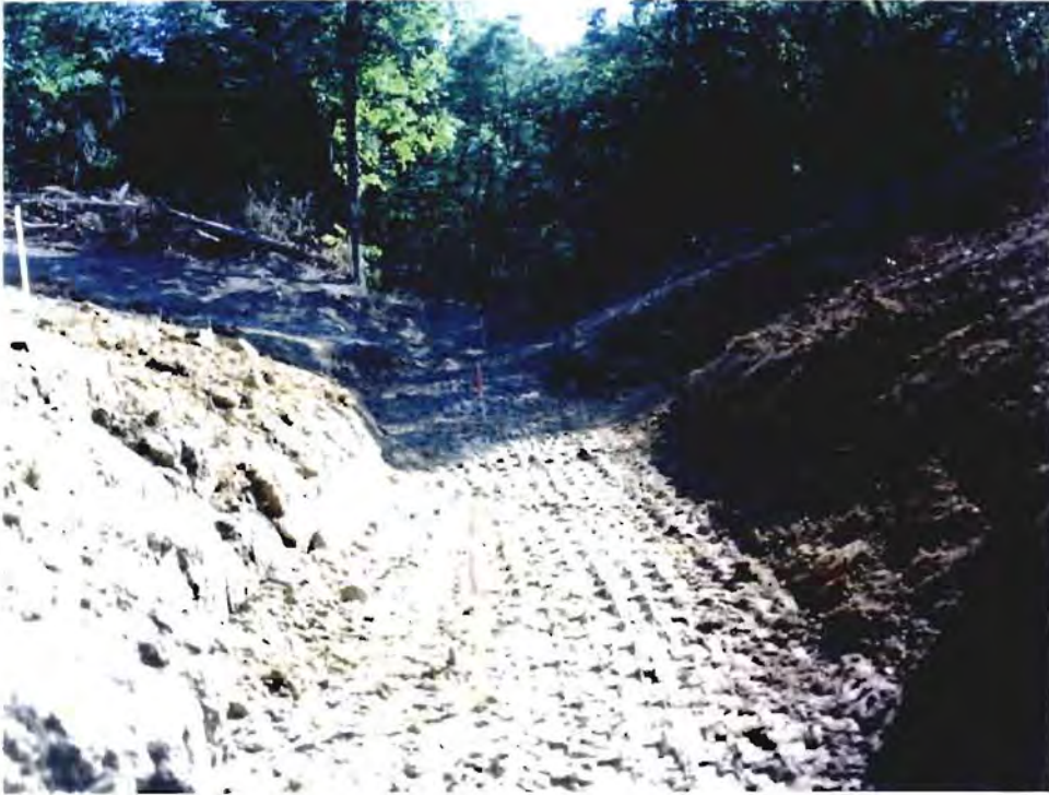
Photo No. 1: (15-16 July 1996) Excavation of the outlet works foundation for the CAMU Sediment Dam. Perpendicular to the excavation is the foundation inspection trench, located along the centerline of the dam alignment.
