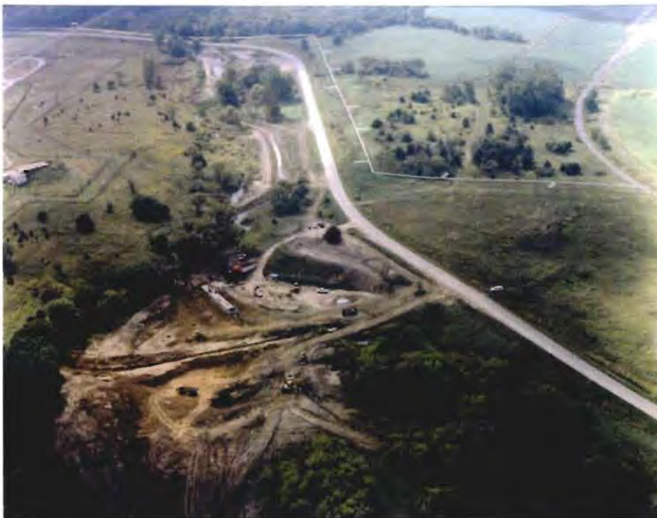
Photo No. 6: (17-18 September 1996) Aerial view of the Wetland Borrow Area. The stilling basin is being constructed and excavation of borrow material is underway.
