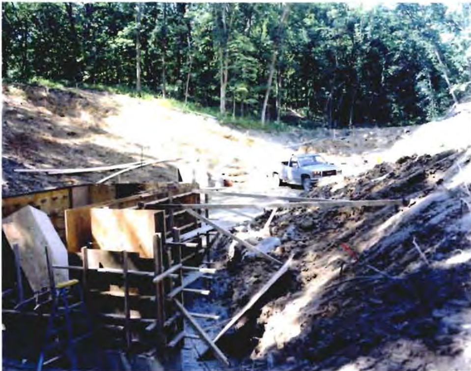
Photo No. 5: (15-16 July 1996) Forms for the reinforced concrete stilling basin are being constructed. The truck is parked at the approximate location of the embankment centerline.
