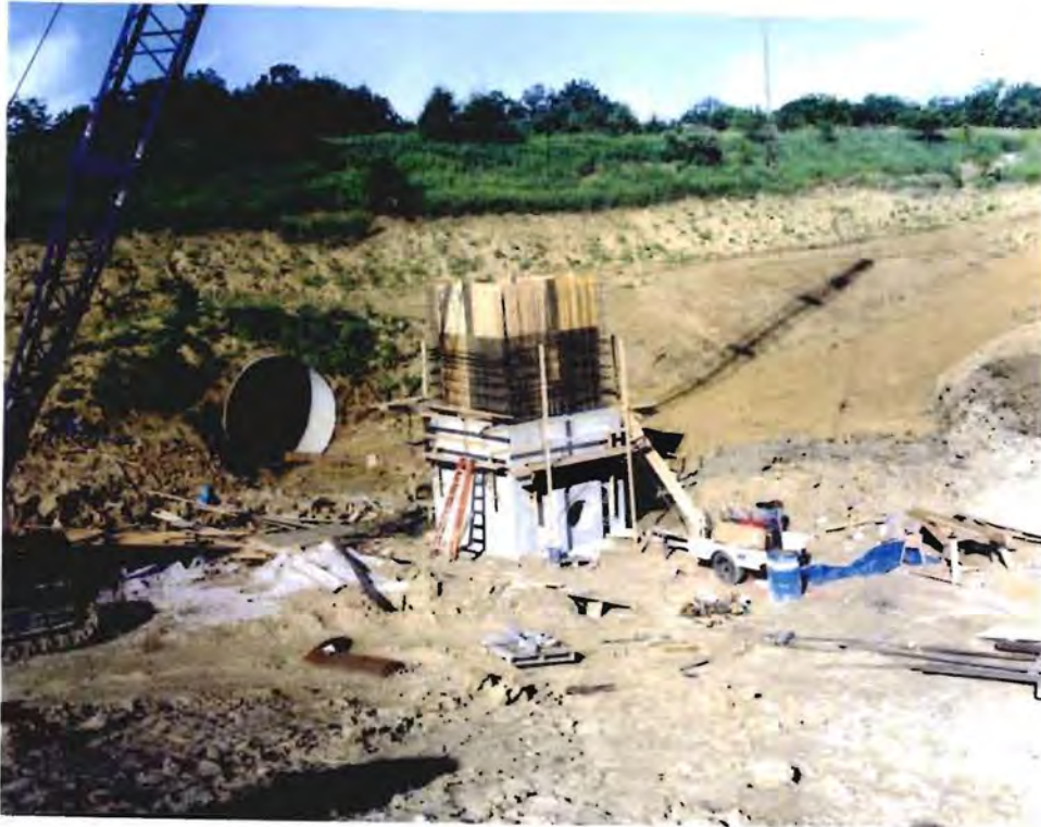
Photo No. 9: (26 June 1997) The new intake structure is under construction. Also visible is the 14 foot diameter conduit through the railroad embankment, and the right abutment inspection trench, located to the right of the intake structure.
