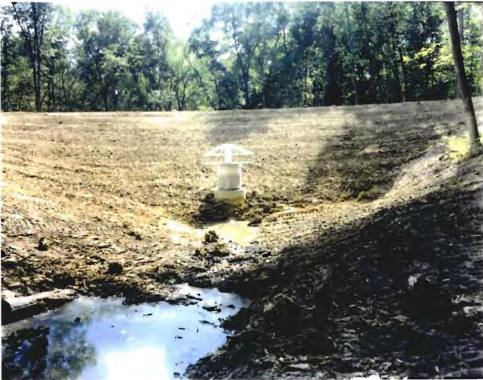
Photo No 8: (17-18 September 1996) View of the intake structure and upstream side of the embankment.
