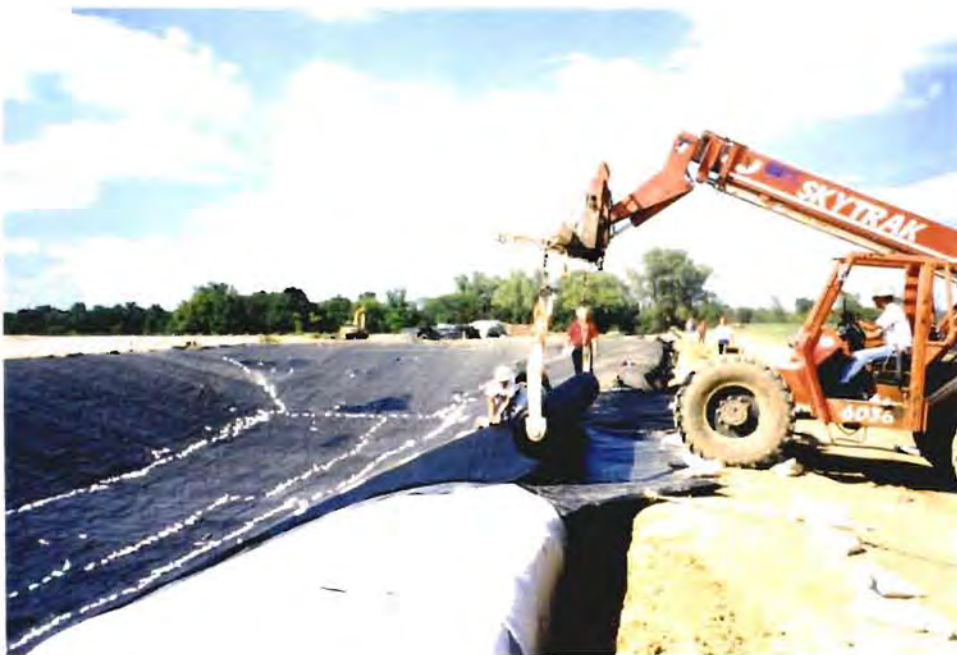
Photo No. 8: (September 1996) View of the geosynthetic anchor trench along the east side of Trench 6, looking north.
