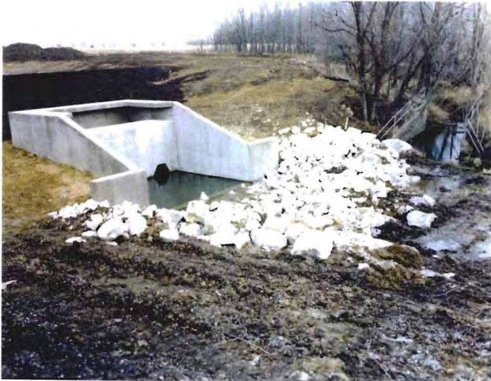
Photo No. 7: (19 November 1996) The stilling basin, and the remainder of the outlet works, is completed.
