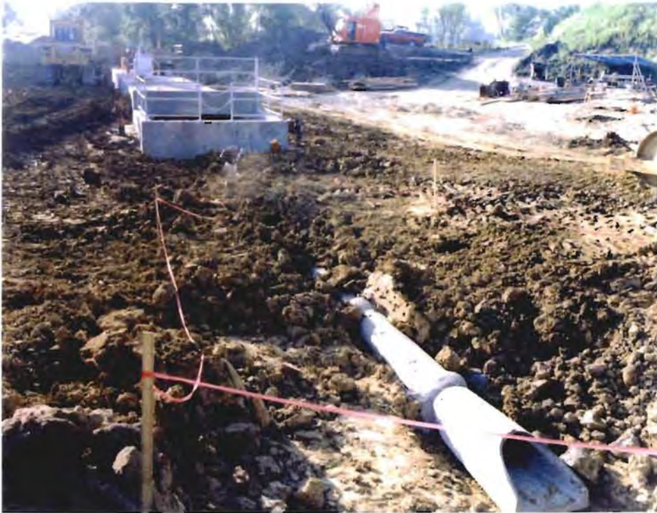
Photo No. 5: (17-18 September 1996) View of the low level intake and intake structure from the reservoir area, prior to final grading.
