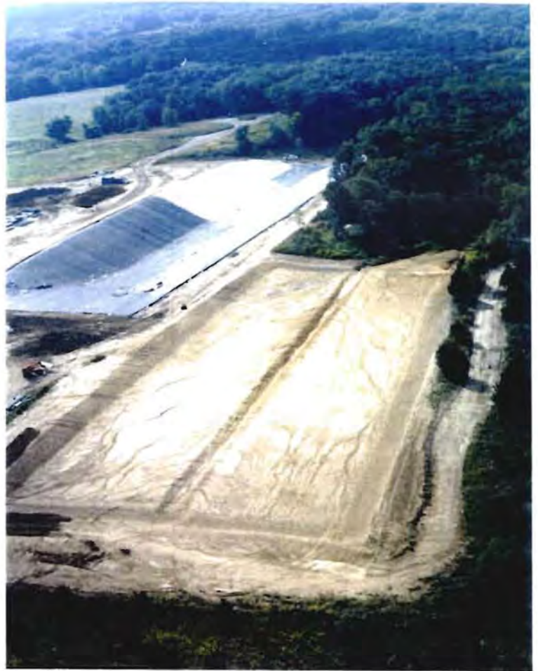
Photo No. 4: (17-18 Sept 1996) Looking southeast at the CAMU foundation preparation and the Trench 6 Soils Repository under construction at the IDA.
