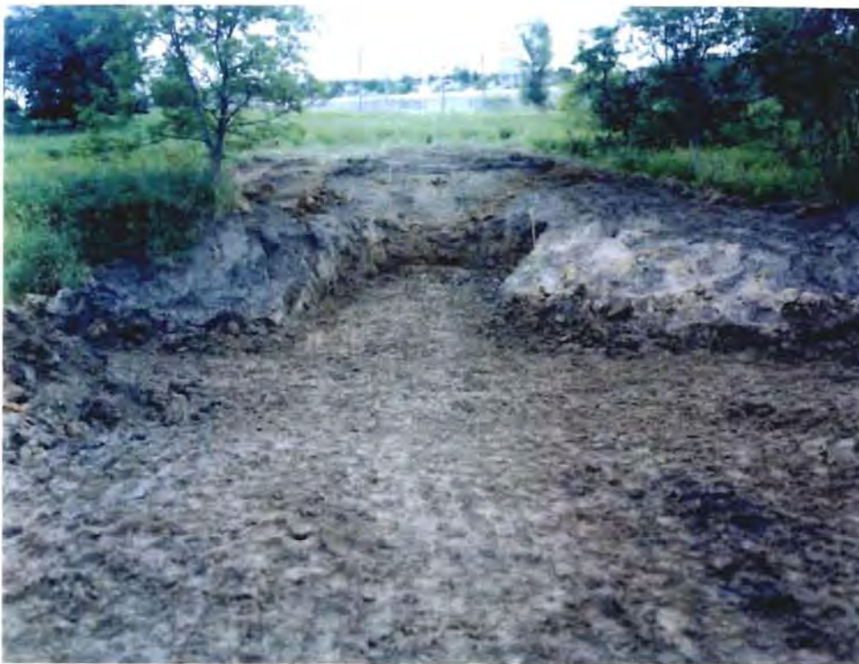
Photo No. 11: (15-16 July 1996) Looking northeast at the cutoff trench and outlet works foundation for the upstream wetlands hydraulic control structure.
