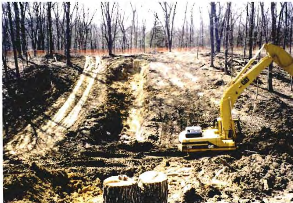
Photo No. 4: (March 1996) Clearing is complete and excavation of the outlet works foundation is in progress. The excavation for the inspection trench in the west abutment can be seen in the center of the photo.
