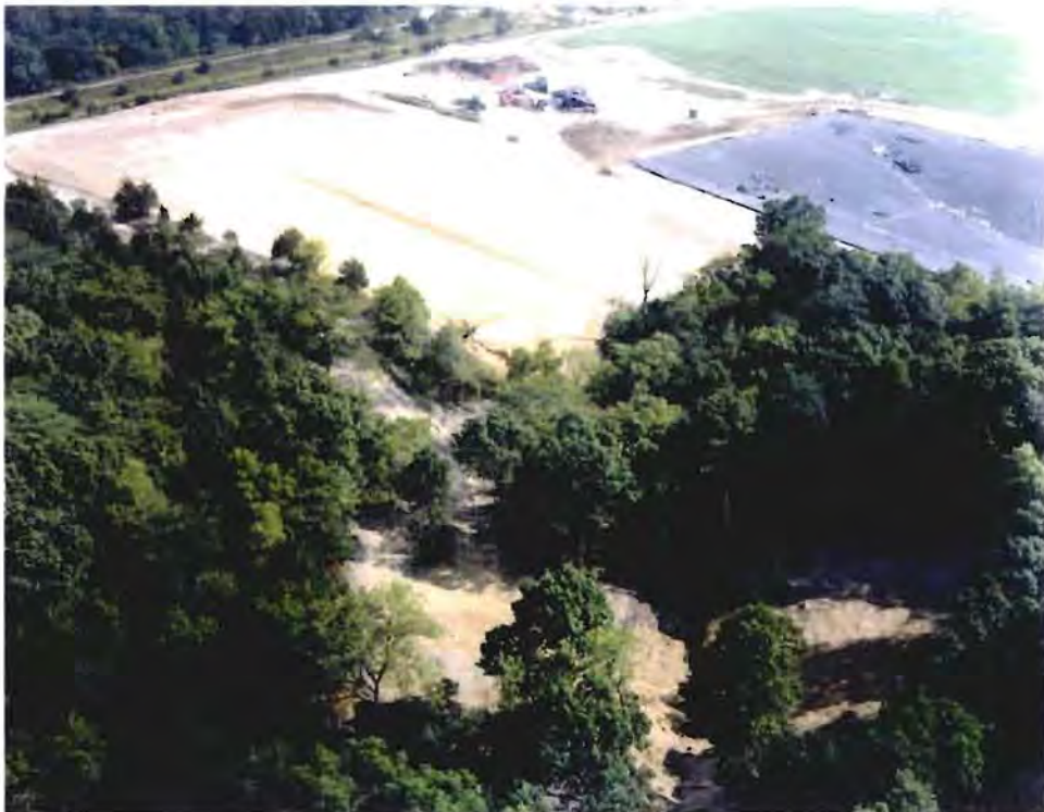
Photo No. 2: (17-18 September 1996) Aerial view of the future location of the CAMU Sediment Dam. The outlet works foundation is visible at the bottom-center of this photo. The CAMU site and Trench 6 are shown above.
