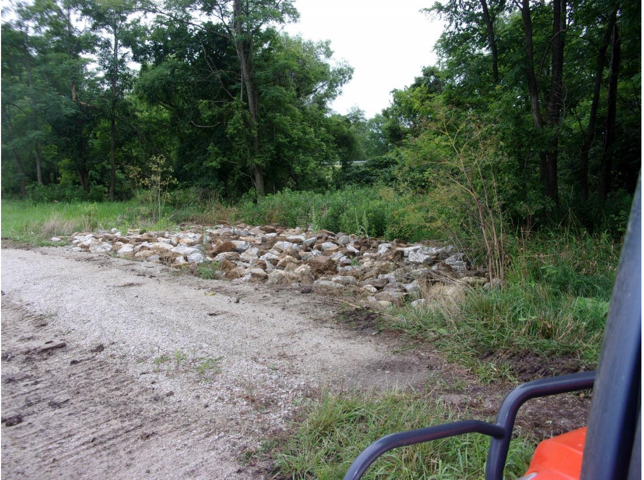
Line 1 Impoundment emergency overflow (August 2021).
