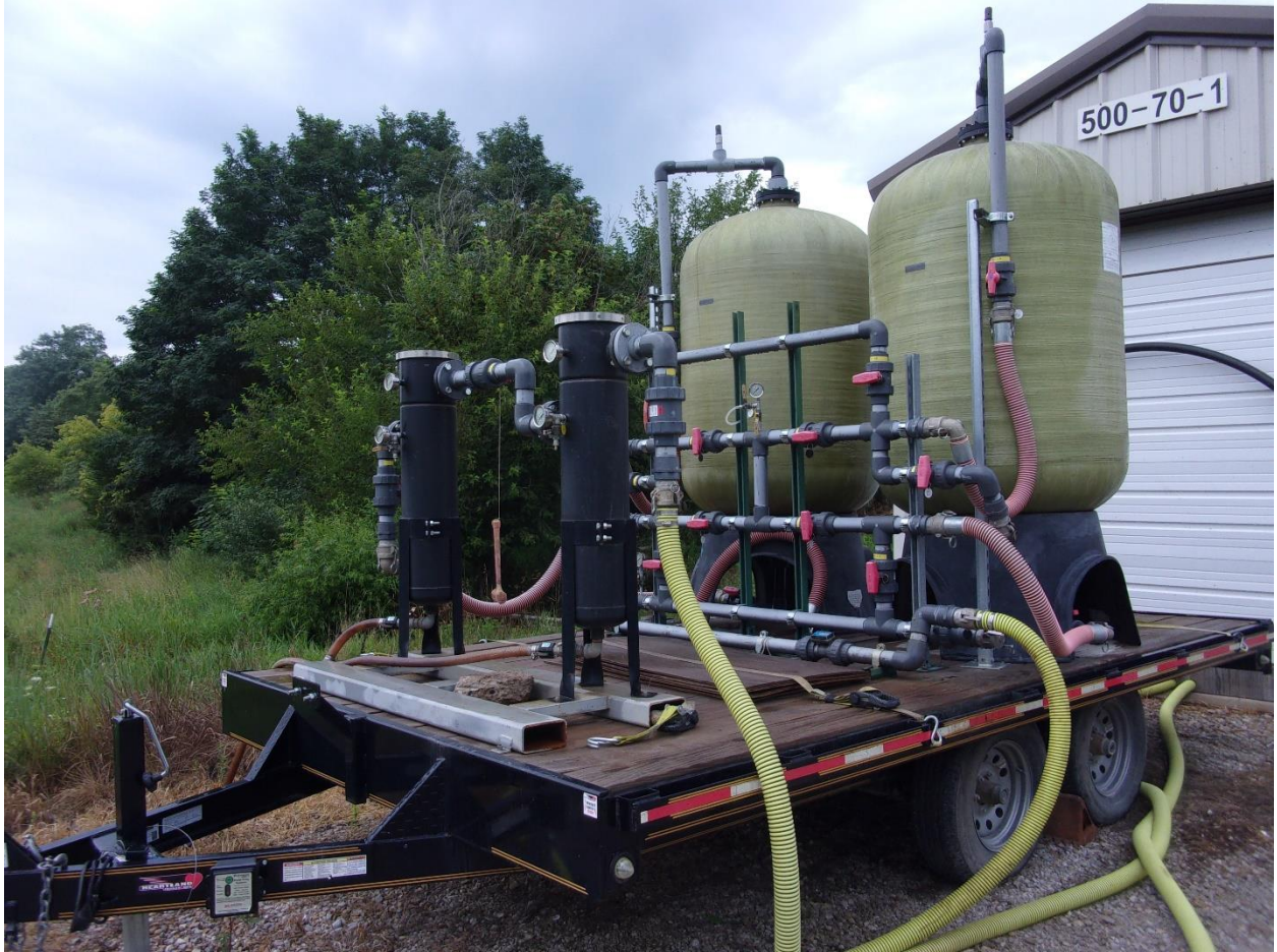
Mobile treatment trailer (August 2021).
