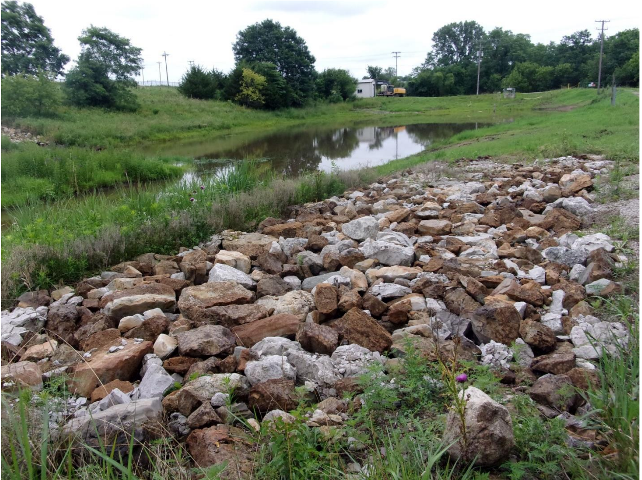
Line 1 Impoundment emergency overflow (August 2021).
