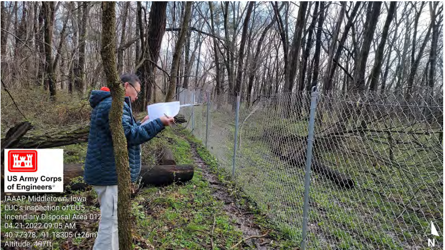
Photo 12 – InDA, Two 10 foot sections of damaged fence (Total of 20 feet fence damaged).
