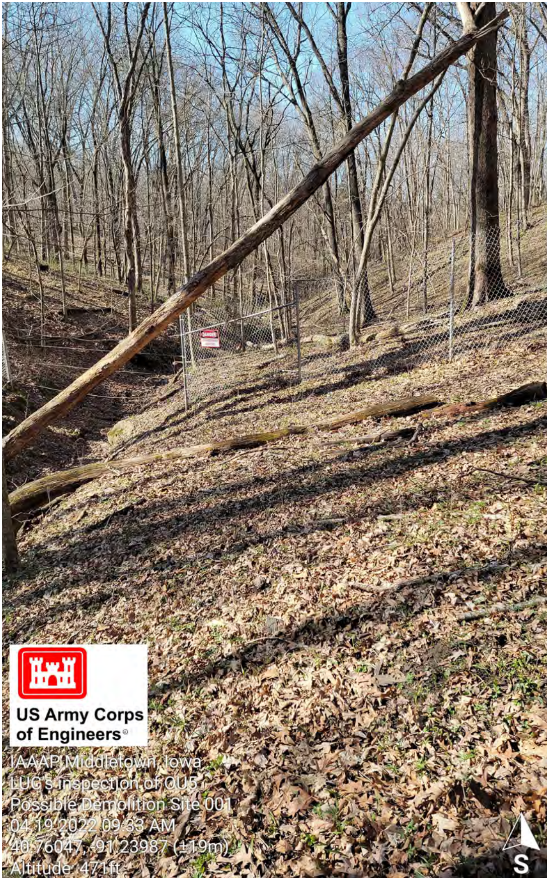
Photo 1 - PDS, Future/potential fence damage (fallen tree).
