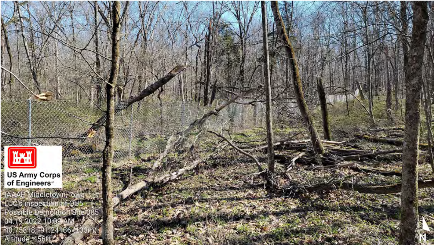
. Photo 5 – PDS, Two 10 foot sections of damaged fence (Total of 20 feet fence damaged).
