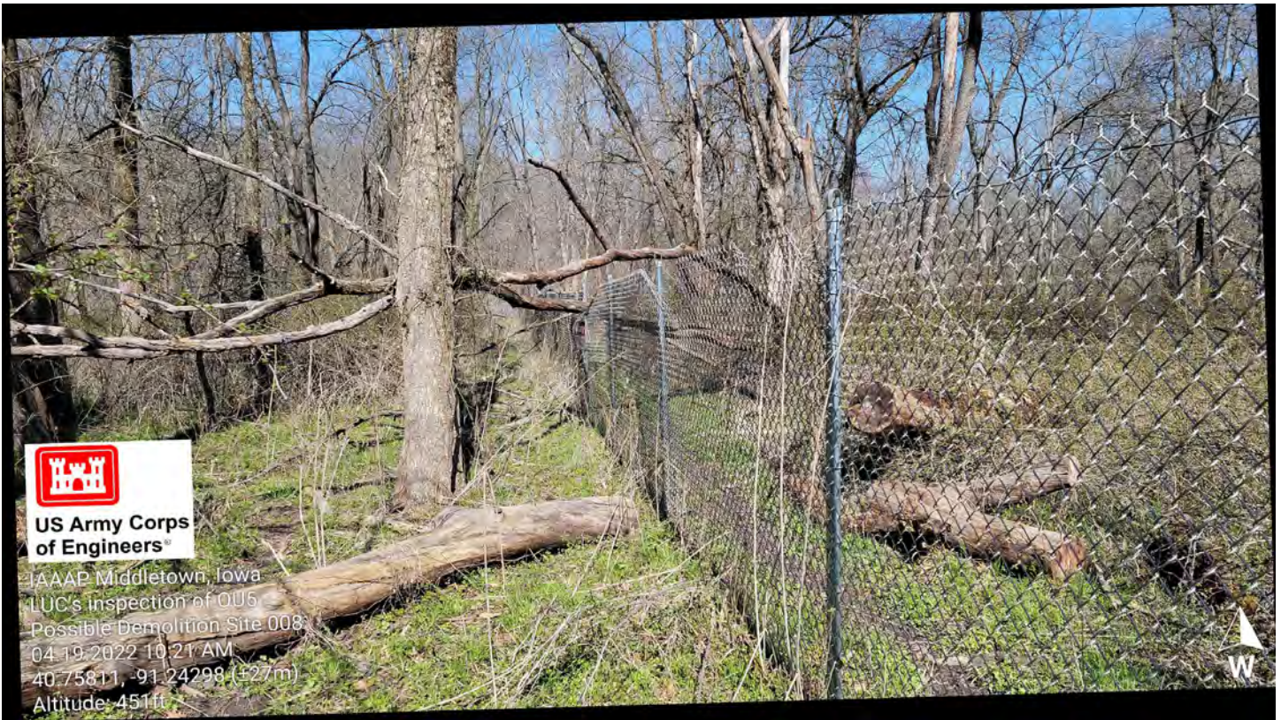
Photo 8– PDS, Approximately 10 feet damaged fence
