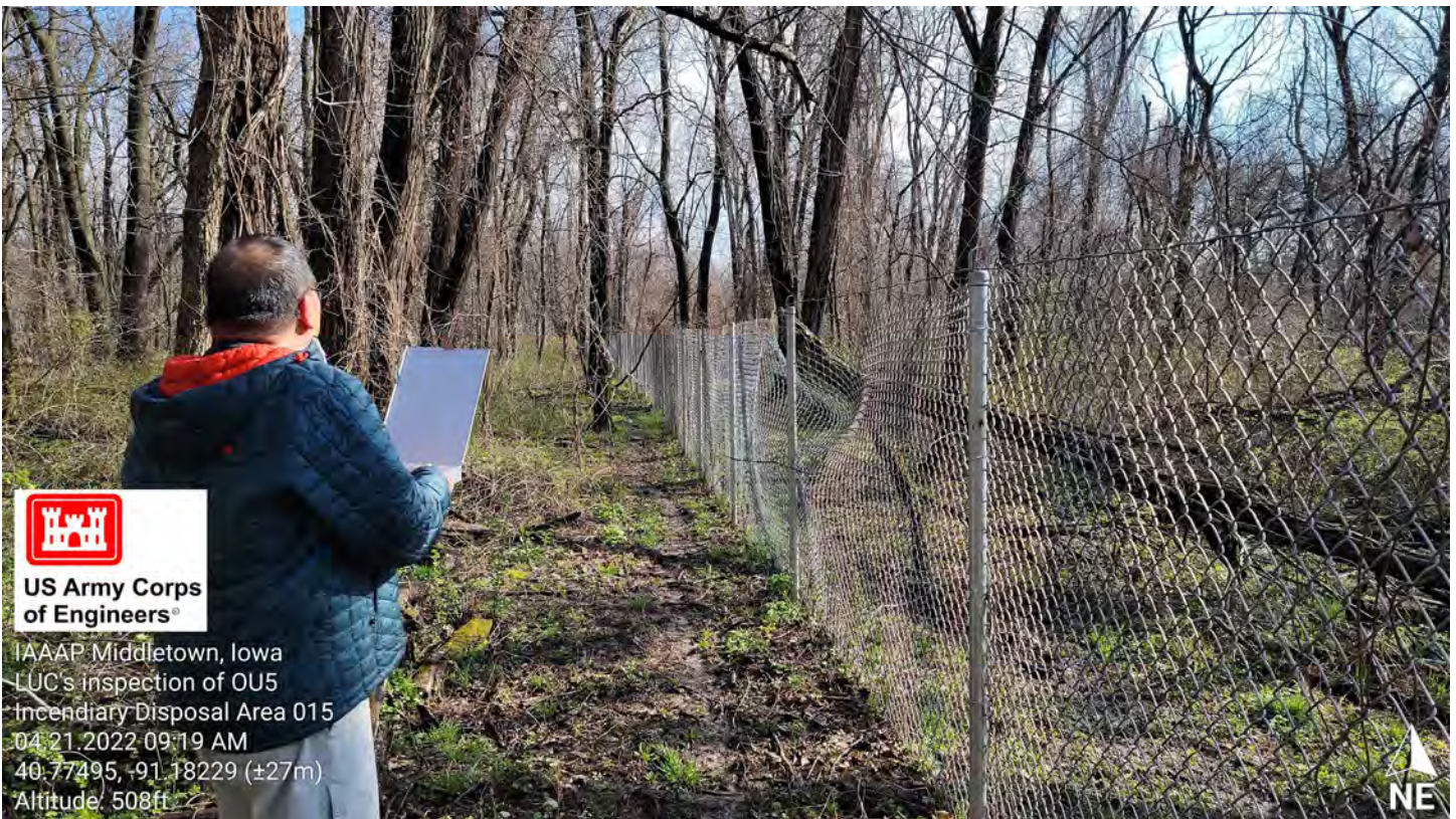
Photo 15 – InDA, 10 foot section of damaged fence.
