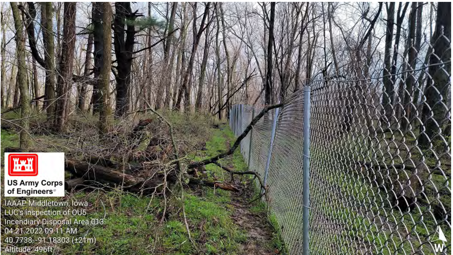
Photo 13 – InDA, Two foot section of damaged fence.
