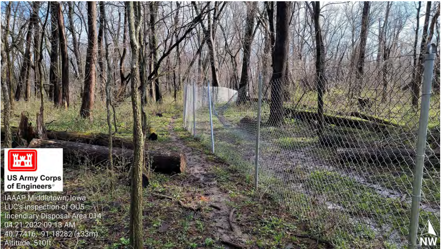
Photo 14 – InDA, 10 foot section of damaged fence.
