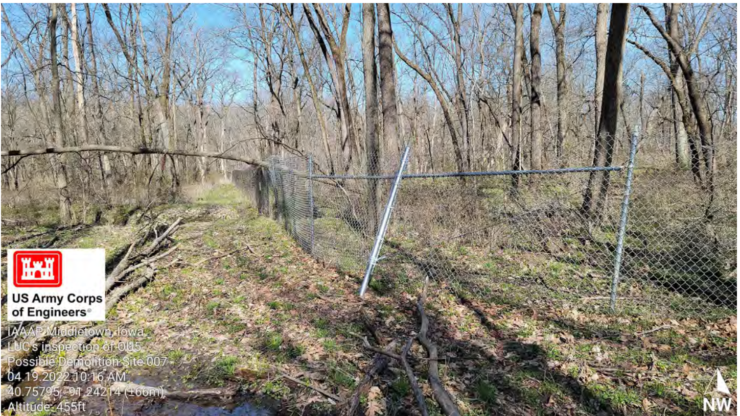
Photo 7– PDS, Approximately 10 feet damaged fence. Post is leaning but stable.
