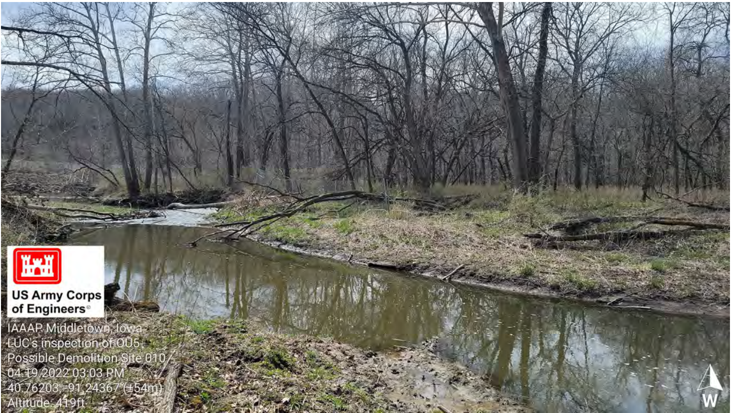
Photo 10– PDS, Approximately 10 feet damaged fence
