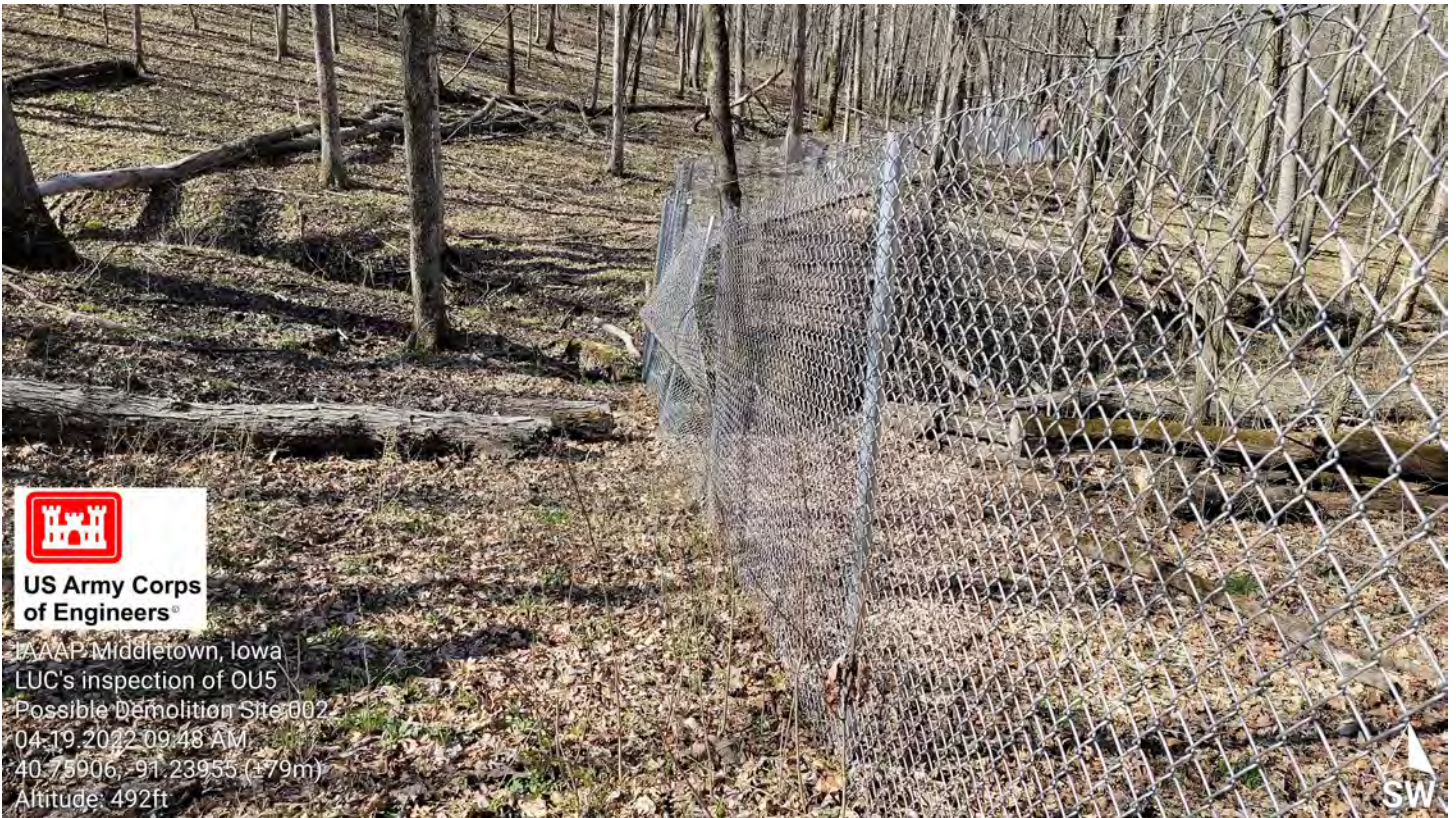
Photo 2 – PDS, Tree has been cut away from fence after damage. Approximately 10 feet damaged fence.
