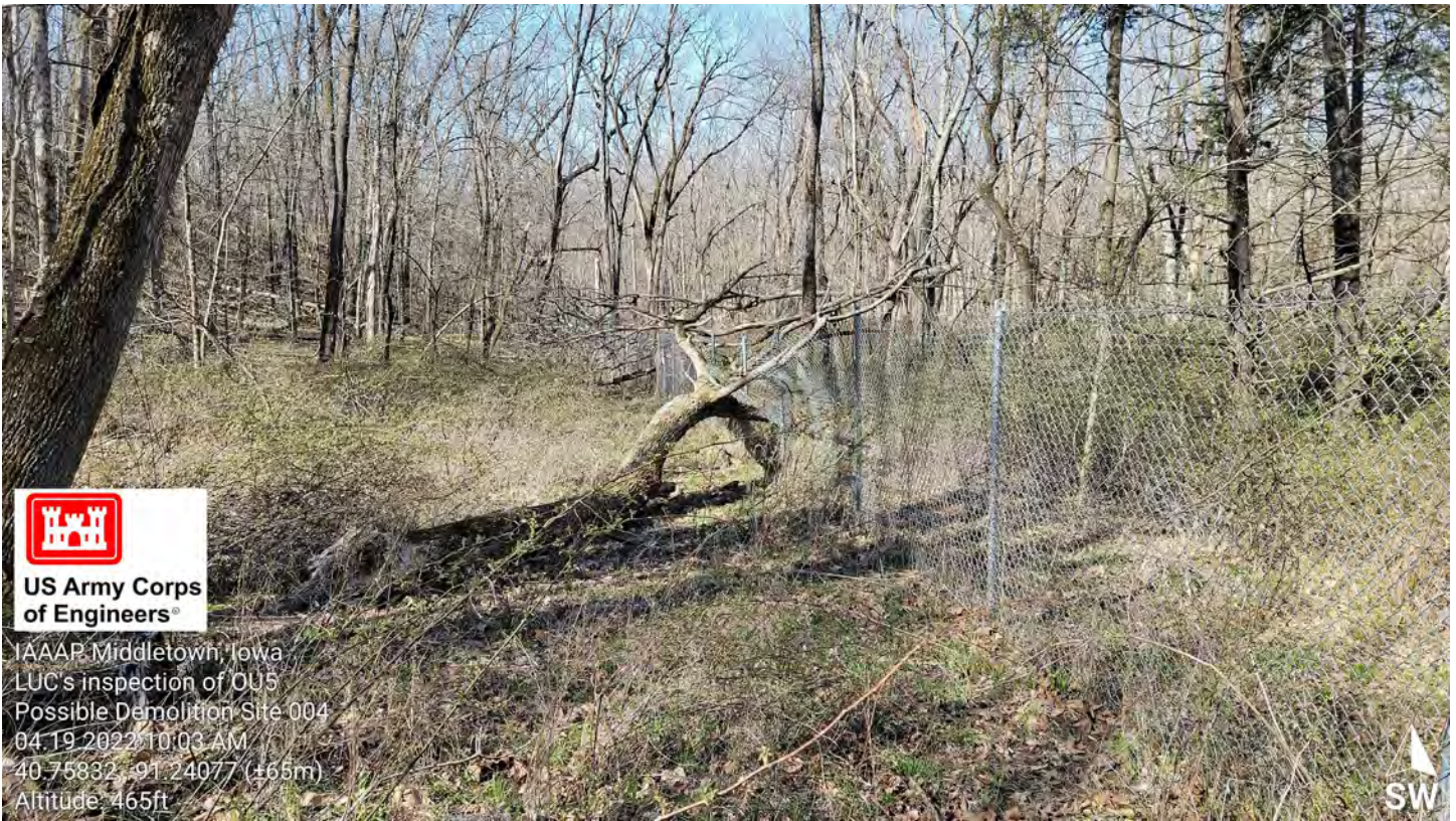
Photo 4 – PDS, Two 10 foot sections of damaged fence, approximately 30 feet apart. (Total of 20 feet fence damaged).
