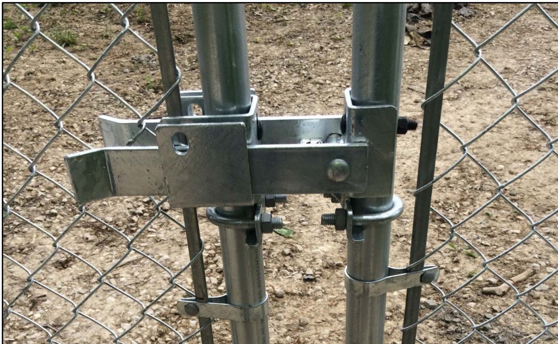
Photo 10. Latch mechanism at Gate #5. Mechanism is the same at all installed double gates.
