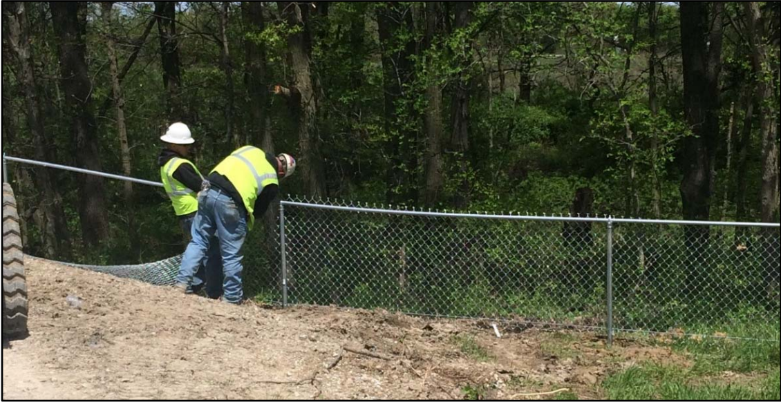
Photo 7. Camera facing west from the west side of trench 6. Attaching the chain link to the frame.
