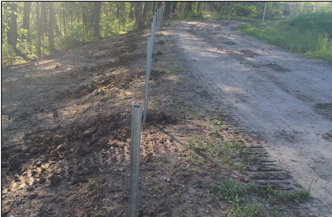
Photo 4. View southeast along access road heading toward the Fixed Facility Water Treatment Plant. Installed fence posts.
