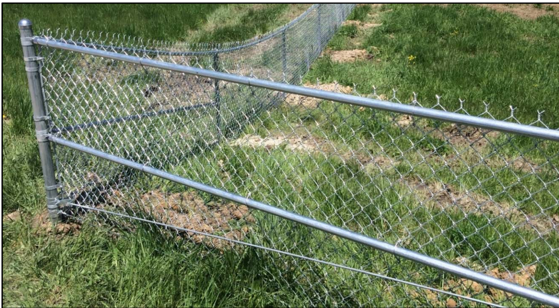
Photo 8. Camera facing north from the east side of the IDA. Showing corner section of fencing with larger end/corner post, tie wire, truss rod, and brace band supplying necessary reinforcement.
