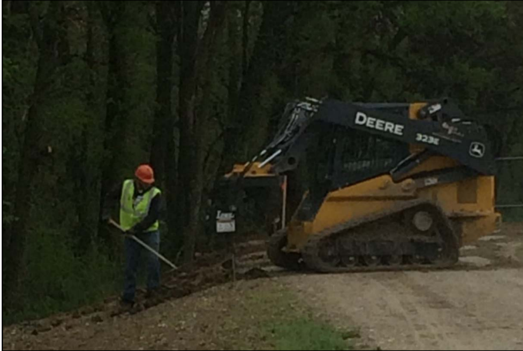
Photo 1. View southwest of the access road toward the Fixed Facility Water Treatment Plant. Skid steer using 12-inch auger to advance fence post holes.
