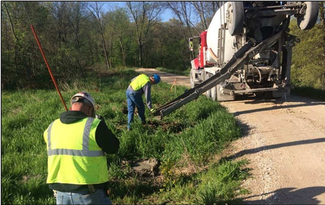
Photo 3. View south along access road heading toward the IDA office. Concrete truck filling the fence post holes with concrete.
