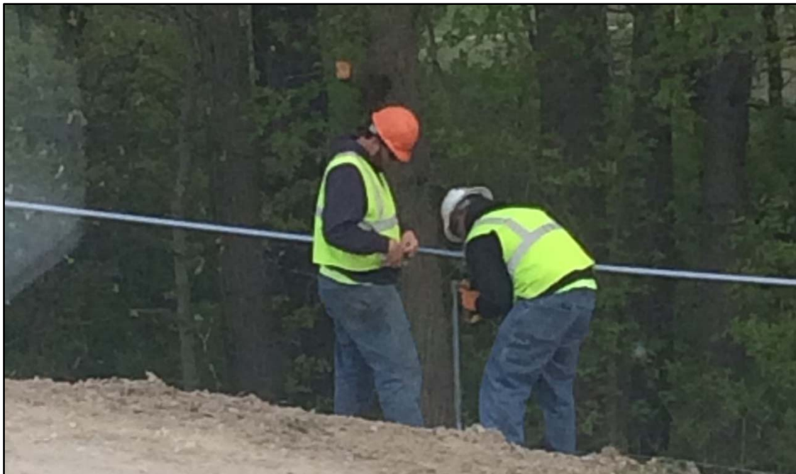
Photo 6. View west along access road to the IDA office. Installation of the fence top bar.
